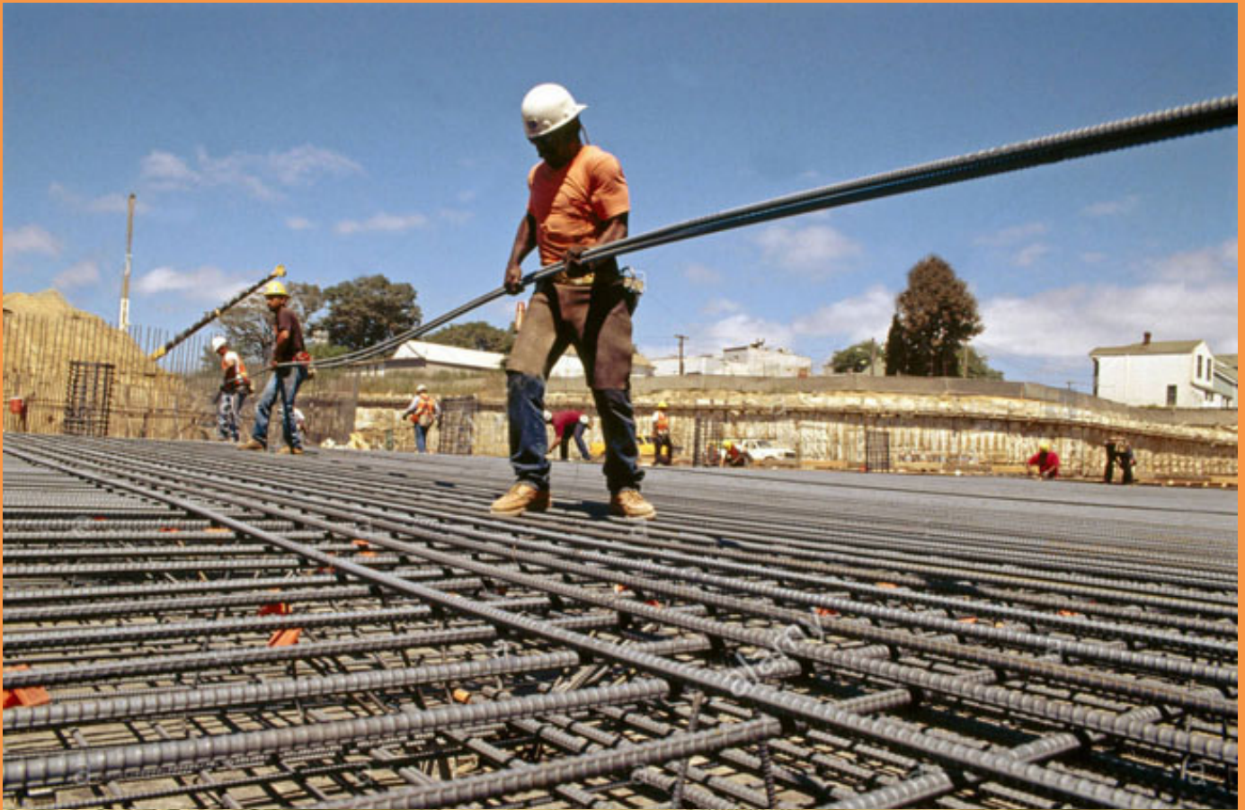
Four "big dumb white guys with pliers", placing 1/2" rebars every 8" or 16" (depending on the job). They're working on the 710 Freeway in Los Angeles. Looks easy, but 30 ft. straight up is the foreman yelling "next bar, move, Move, MOVE!".
