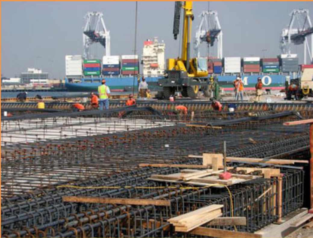
A vast berth of rebar....looks like it's hot out there in the sun!
