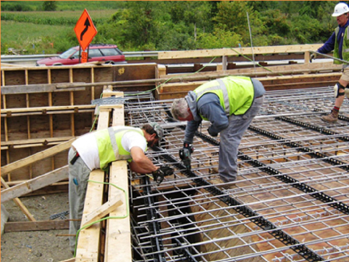
Looks like a bridge deck, but it could have been one of the miles of subway I worked on just west of downtown L.A., perhaps MacArthur Park. Lots of steel on that job. There was a nasty young foreman supervisor, I recall!
