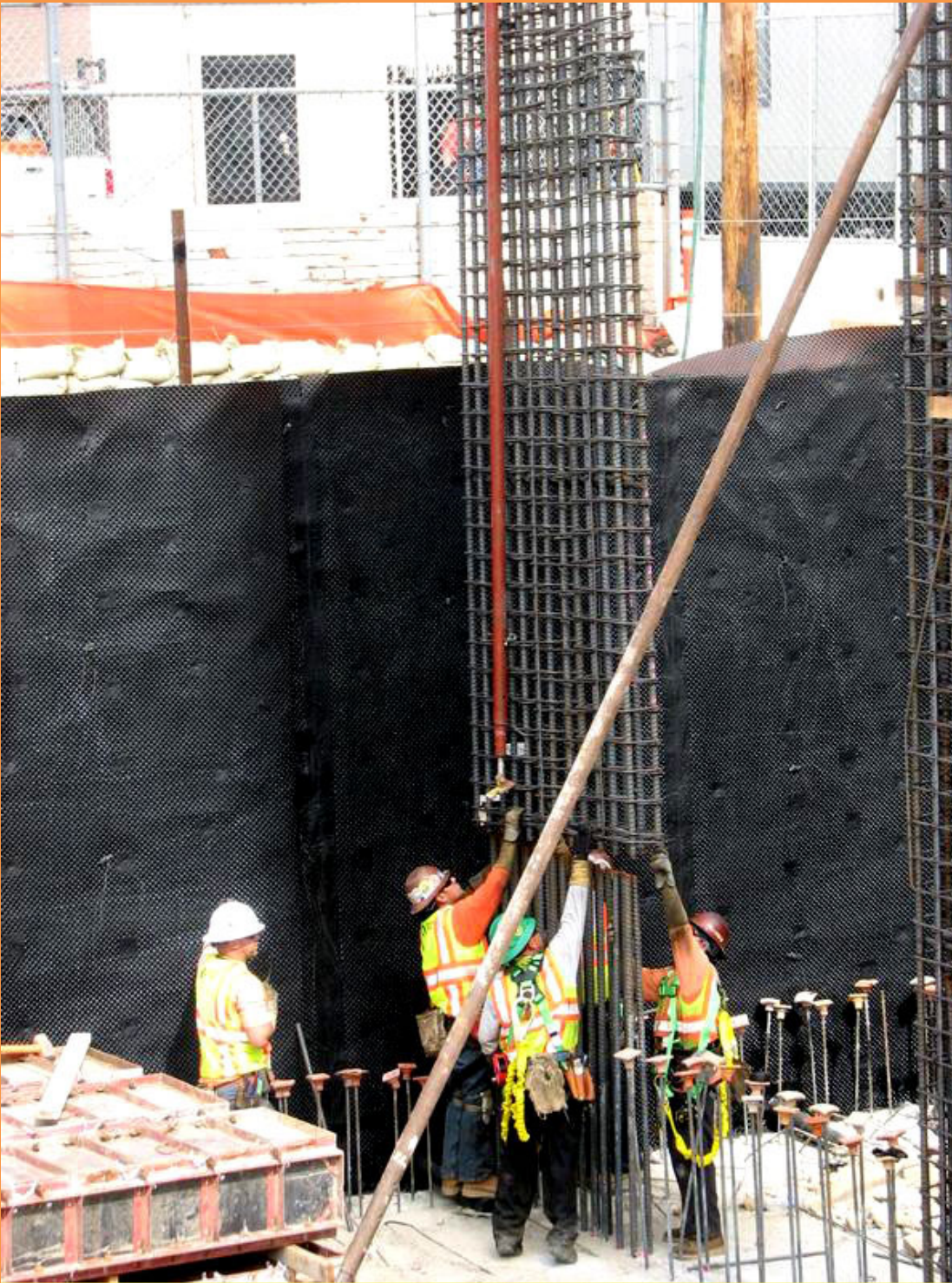
The vertical rebar in this column is usually more than an inch in diameter. This support column could be used for the foundation of a building, a parking lot, or whatever the blueprint specifies. We often were not told what kind of project we were working on - remember, we were just "big, dumb white guys"!
