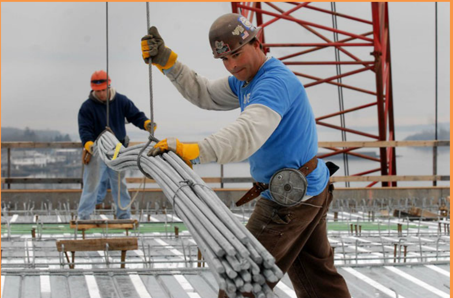
These guys were lucky - they have a hoist. I used to carry bundles of rebar like this on my shoulder....
